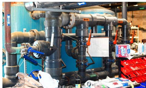
Mechanical pool plumbing
