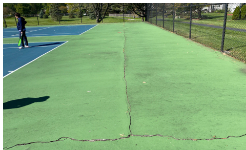
Cracks in tennis courts
