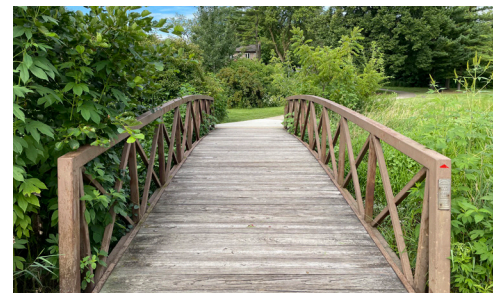
Pedestrian bridge in need of maintenance
