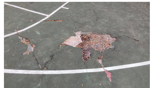
Spalling concrete at basketball court
