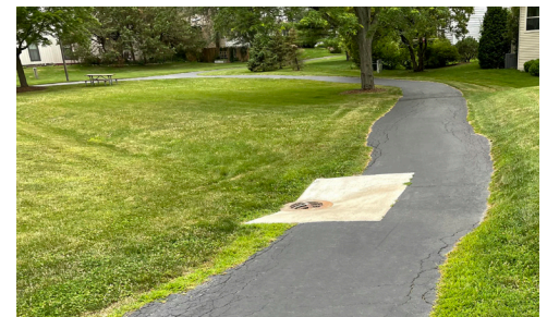
Drainage swale and inlet
